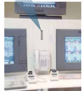
SIS Indicator in control room.
