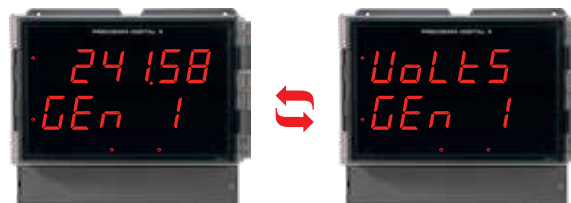
Upper line toggles between 241.58 and Volts and the lower line displays Gen 1
